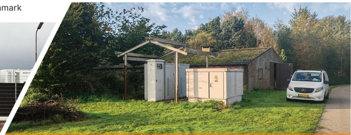
200kW/465.92kWh Microgrid System
