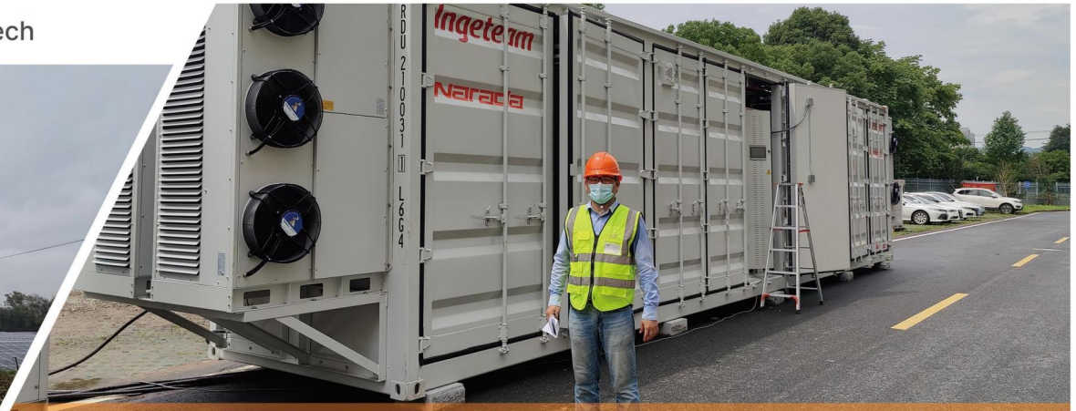
70MWh BESS System in Hangzhou, Zhejiang
